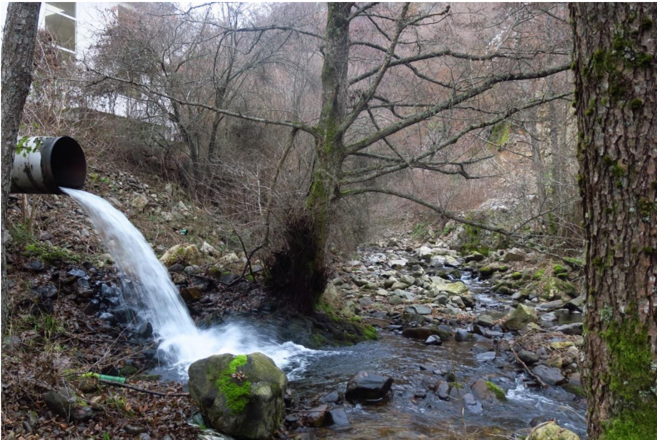
Discharge of water below Blagoevgradska Bistritsa-8 HPP not described in the EIA/AA screening decision, 21 December 2020
